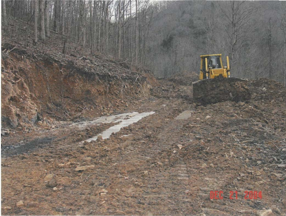
Photograph 7 Maintaining the Site after a Bank Slip
